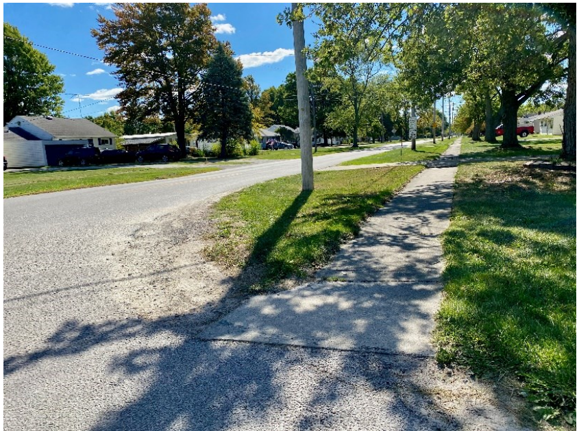
Gap in sidewalk connectivity on Townline and North Benton St. near Oak Harbor High School. October 2024.
