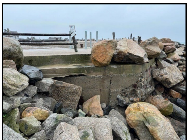
Sakonnet Point Breakwater Storm Damage Photo Credit: Chris Brady
