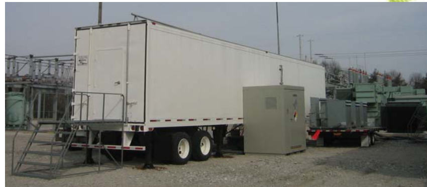
AES 1 MW substation energy storage system
