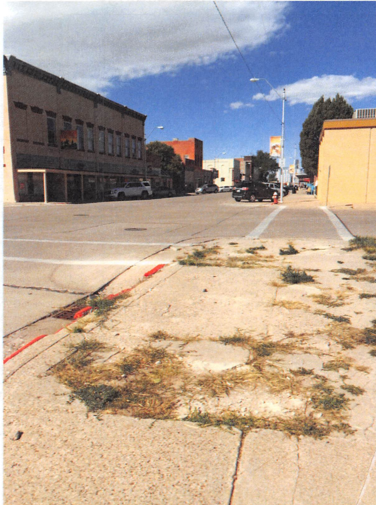
Sidewalk breakup and missing sidewalks not only look unattractive but are a barrier to people accessing the places they want to go if they have limited mobility or rely on wheelchairs or scooters to get around.
